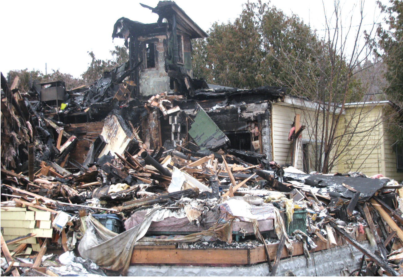
The Charlevoix Hotel at 206 Antrim St. is a total loss from a fire that broke out during the early morning hours on Saturday, Jan. 28. No one was hurt in the fire that started in a bathroom of the 10-room hotel.
